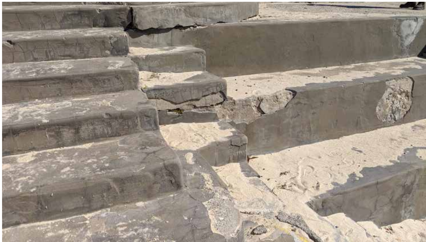
Damaged and unsafe conditions of existing bleachers and stairs
